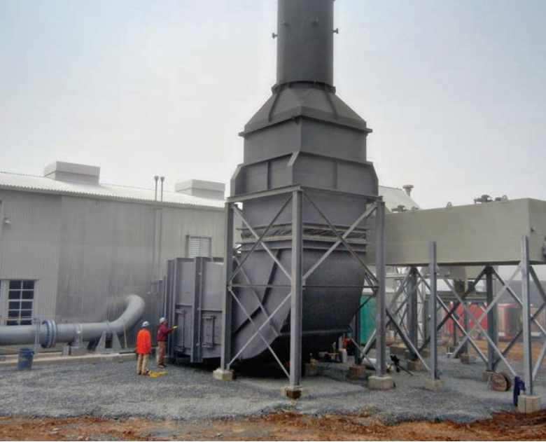
FILTER HOUSE FOR BRUSH GENERATOR
