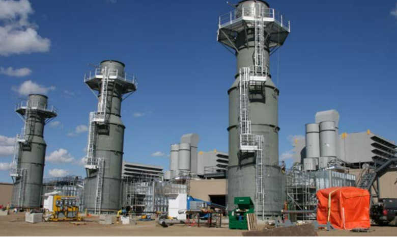
EXHAUST SILENCING SYSTEMS AND ANTI-ICING SYSTEM FOR 3 X GE LM6000
