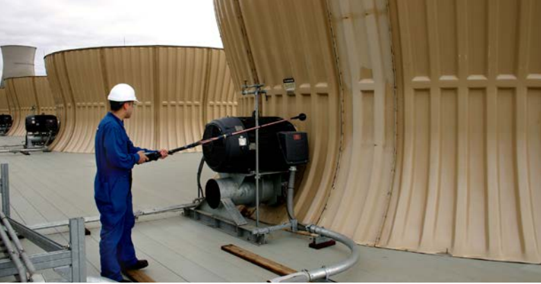
NOISE MEASUREMENTS OF A COOLING TOWER
