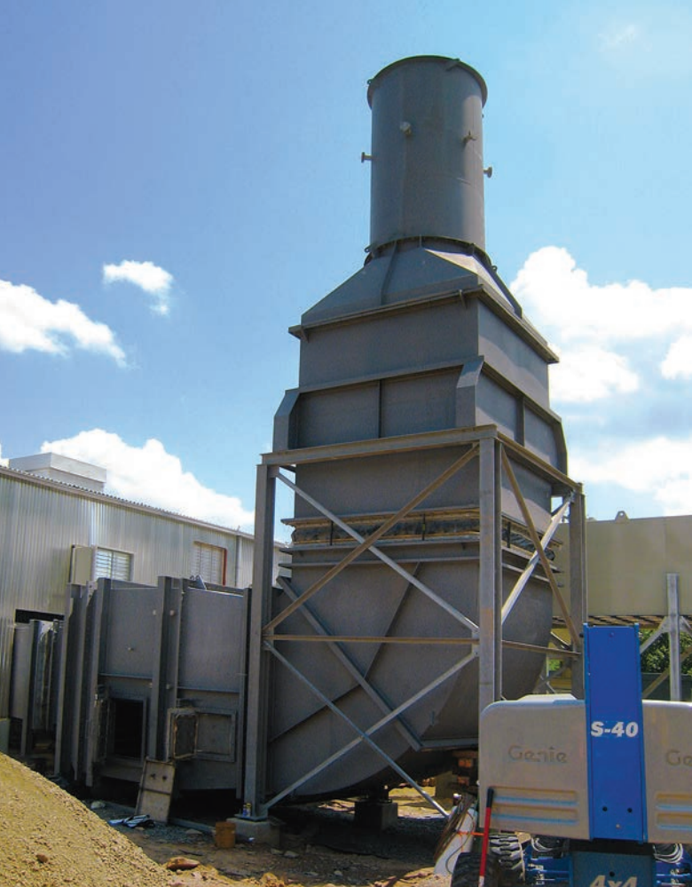
EXHAUST CATALYST AND SILENCER FOR A MARS 100 GAS TURBINE
