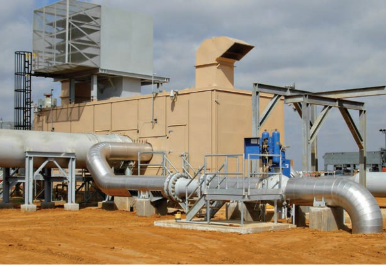
ACOUSTIC ENCLOSURES AT A GAS PLANT IN HOUSTON, TEXAS
