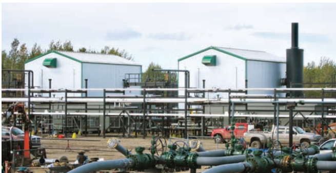
TWO ON-SKID COMPRESSOR STATIONS IN DAWSON CREEK, BC
